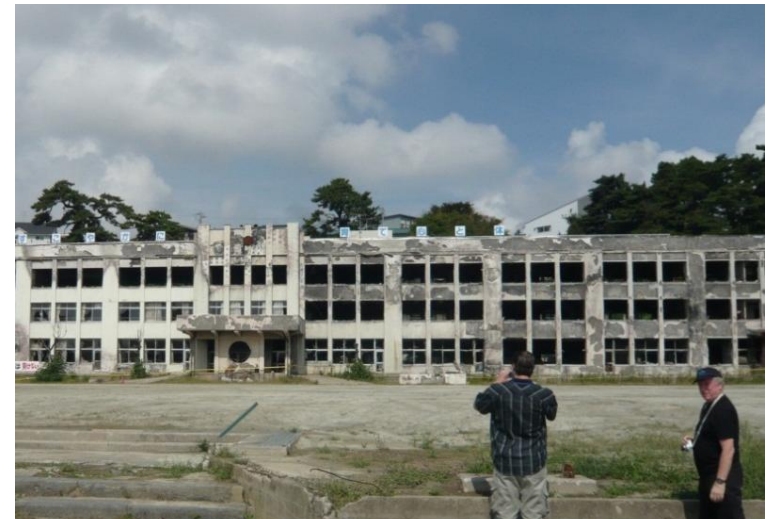
School damaged by 311tsunami
